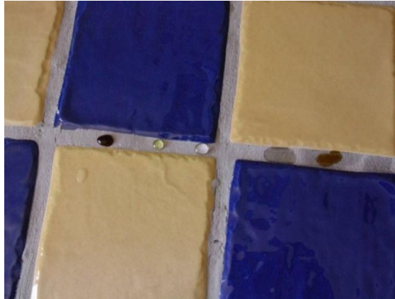
Rys. 4.27. Silne zabrudzenia fug [ https://enamai.lt/lt/statybos-akademija/kaip-priziureti-plyteles ]
